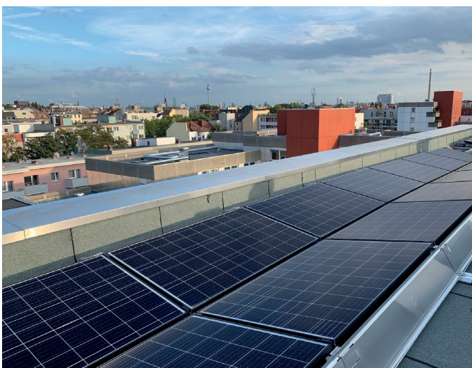
The PV system at Adolfstraße 4, with an output of more than 30 kWp, comprises over 100 modules. (photo)
